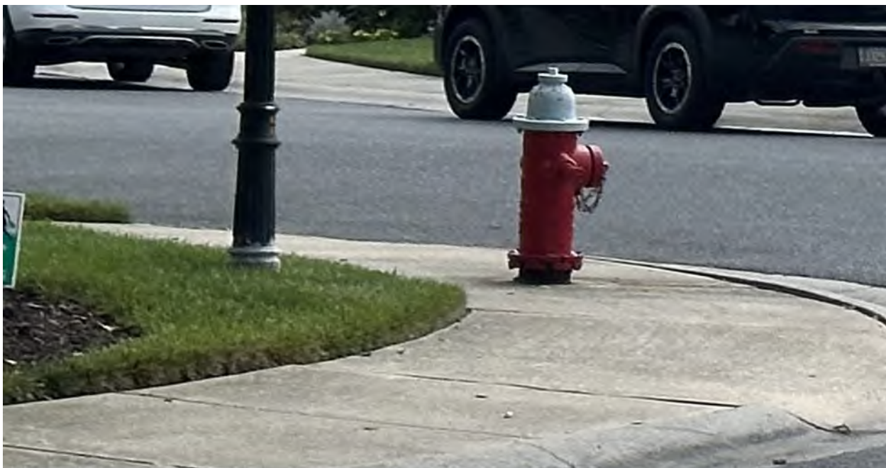
Figure 12 Fire hydrant in sidewalk at NW corner of Cinder Way and Mulberry St
