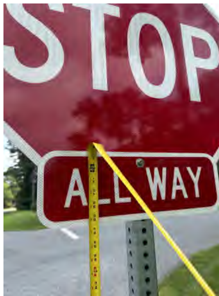
Figure 5 Height of Stop Sign along Cinder Way at the intersection of Boisenberry Ln. Per MUTCD, the bottom of the Stop Sign must be at least seven feet above the near edge of the travel way, and the secondary sign may be one foot less in height.
